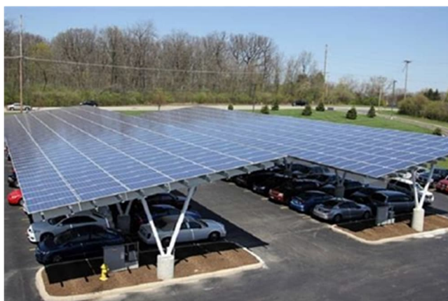
Figure 9: Example of a solar PV carport with steel support structure
